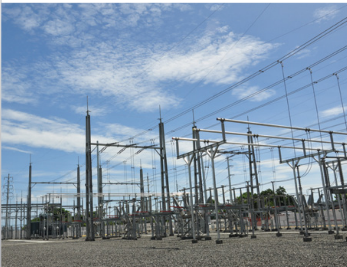
Visayan Electric Company Inc. (VECO) Naga 138 kV Switchyard
