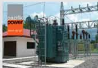
Design, construction and energization of substation up to 100MVA (PPI Pazifik Power, Inc., Philippines)
