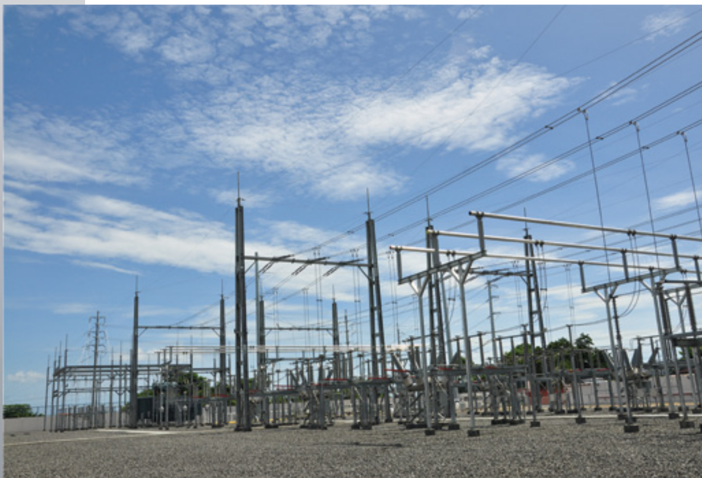
VISAYAN ELECTRIC COMPANY INC. (VECO) NAGA 138KV SWITCHYARD
